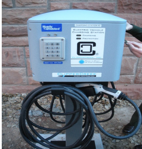
Figure 8. Non-networked EV charging station at Zion National Park, utilizing a keypad payment method. Codes are sold at park visitor centers at a set price.
