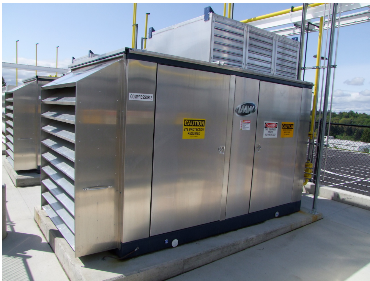
Figure 30. Two compressors at a CNG station
