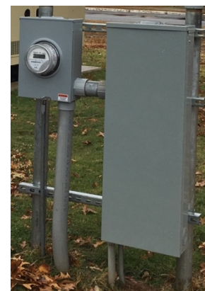
Figure 20. Meter and panel
