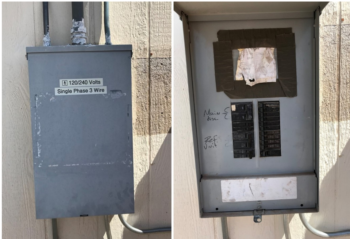
Figure 16. Single-phase service panel at Fort Bliss
