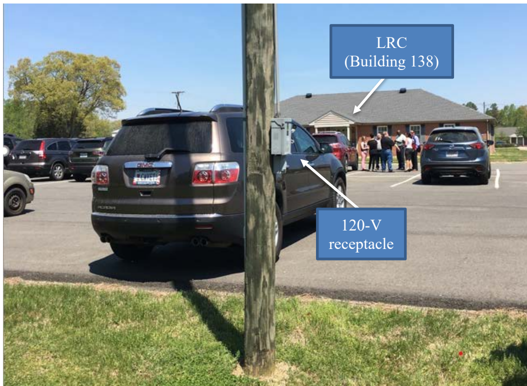
Figure 24. Level 1 receptacle at Fort A.P. Hill
