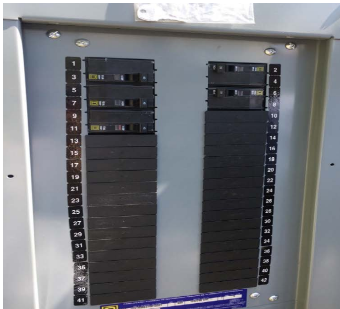
Figure 18. Service panel at Fort Myer-Henderson TMP
