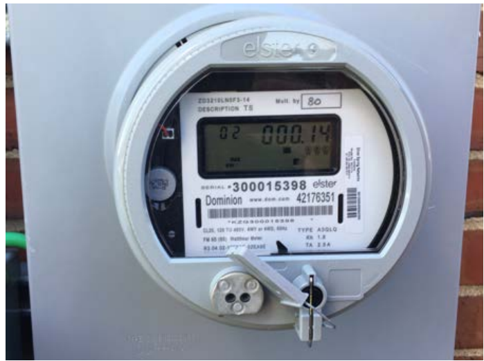
Figure 17. Fort Belvoir power demand meter
