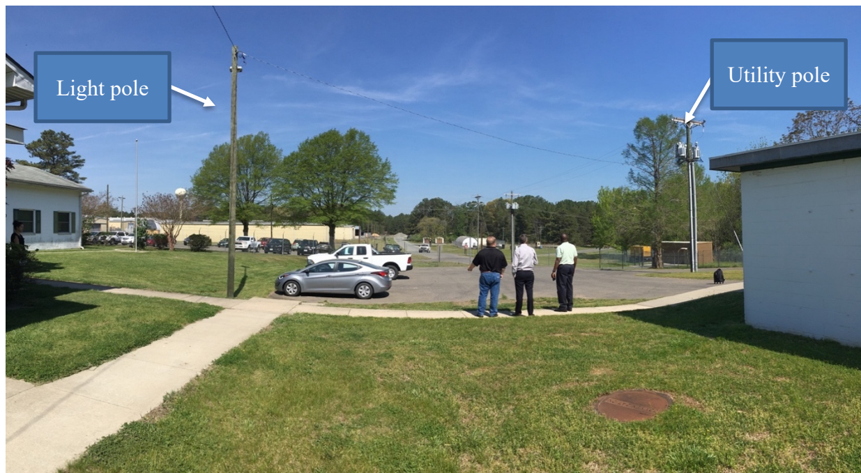
Figure 14. Overhead transformer connection at Fort AP Hill
