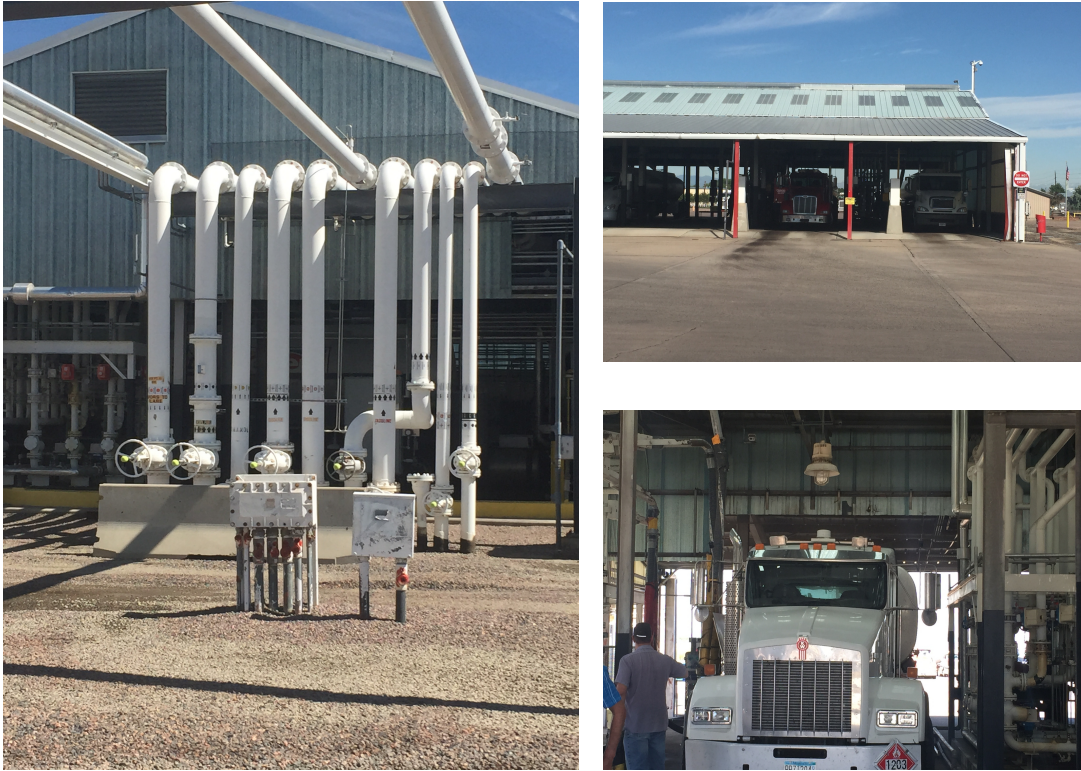
Figure 3. Loading rack and bay
