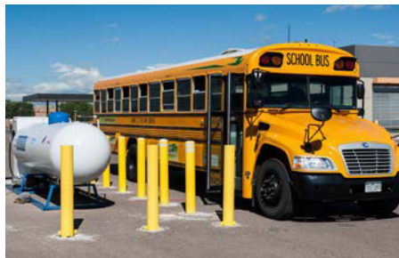
This Colorado school district started with one 1,000-gallon storage tank and later expanded its capacity by adding a second tank. Photo by Dennis Schroeder, NREL 31321.
